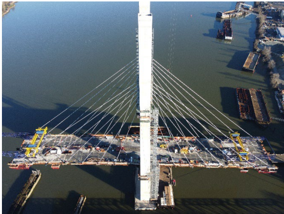
Figure 3: Girder erection, deck panel, and stay cable installation for the main bridge continues. In this photo, 7 pairs of cables are installed on both the south and north side of the tower.
