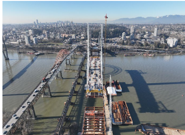
Figure 4: Aerial view of the South Approach shows progress to close the gap between the bridge tower and S2, known as the back span.
