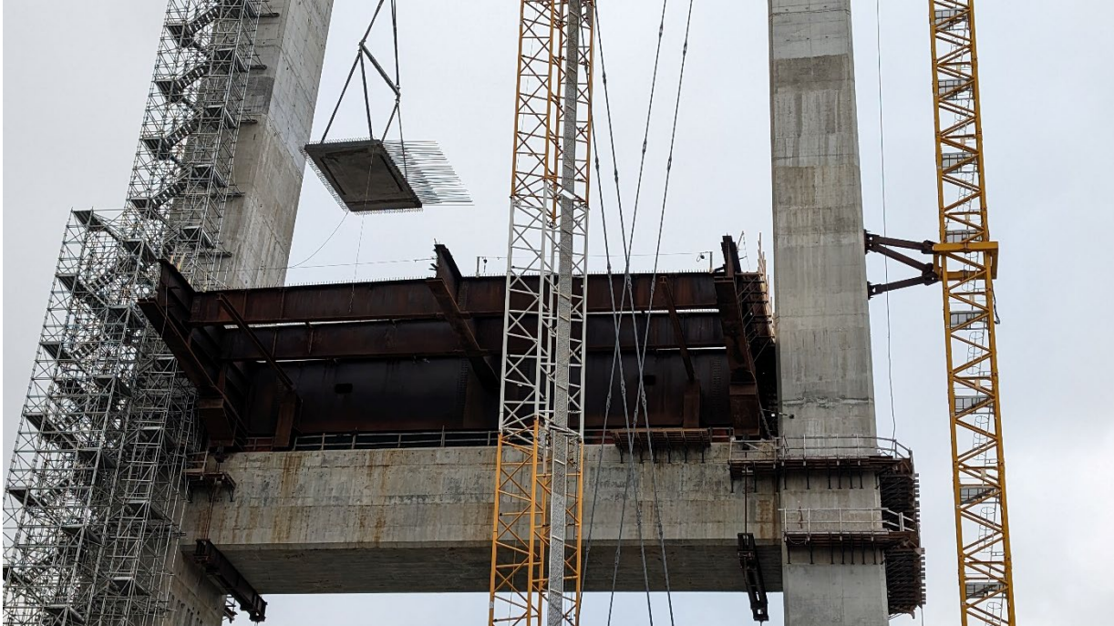
Figure 2 – Crane lifting a precast deck panel onto the bridge tower's lower crossbeam.
