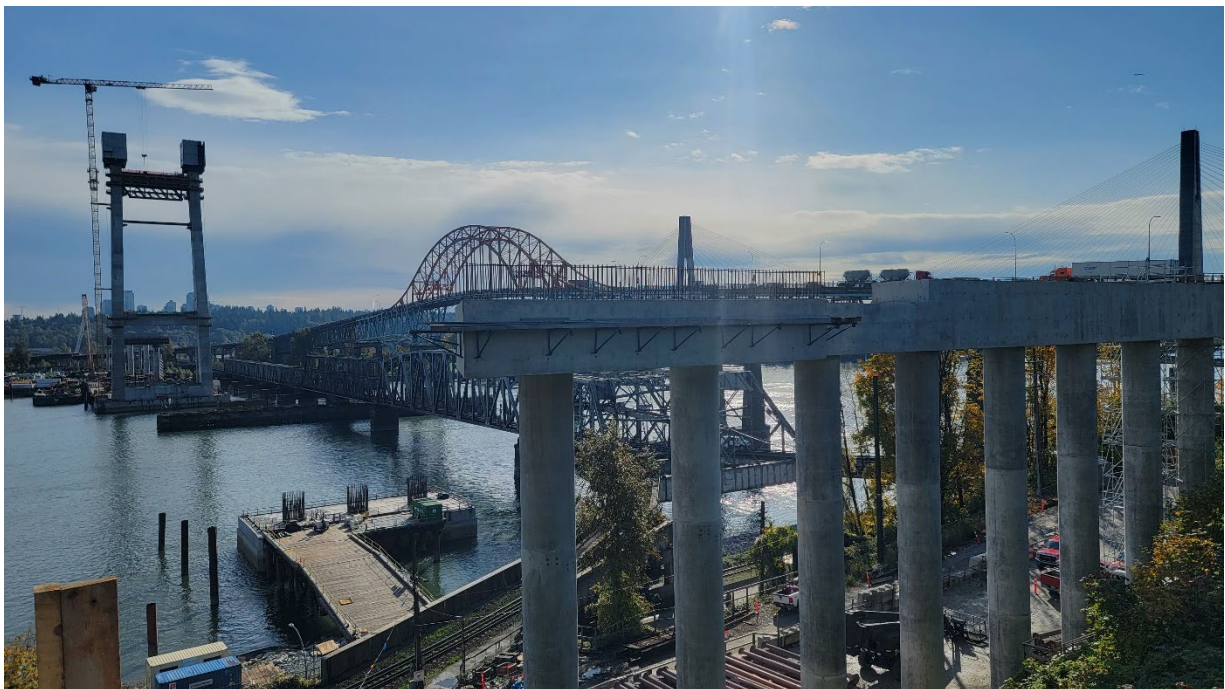
Figure 4 – Pier N2 In New Westminster And The Two In-River Piers N2 And S1
