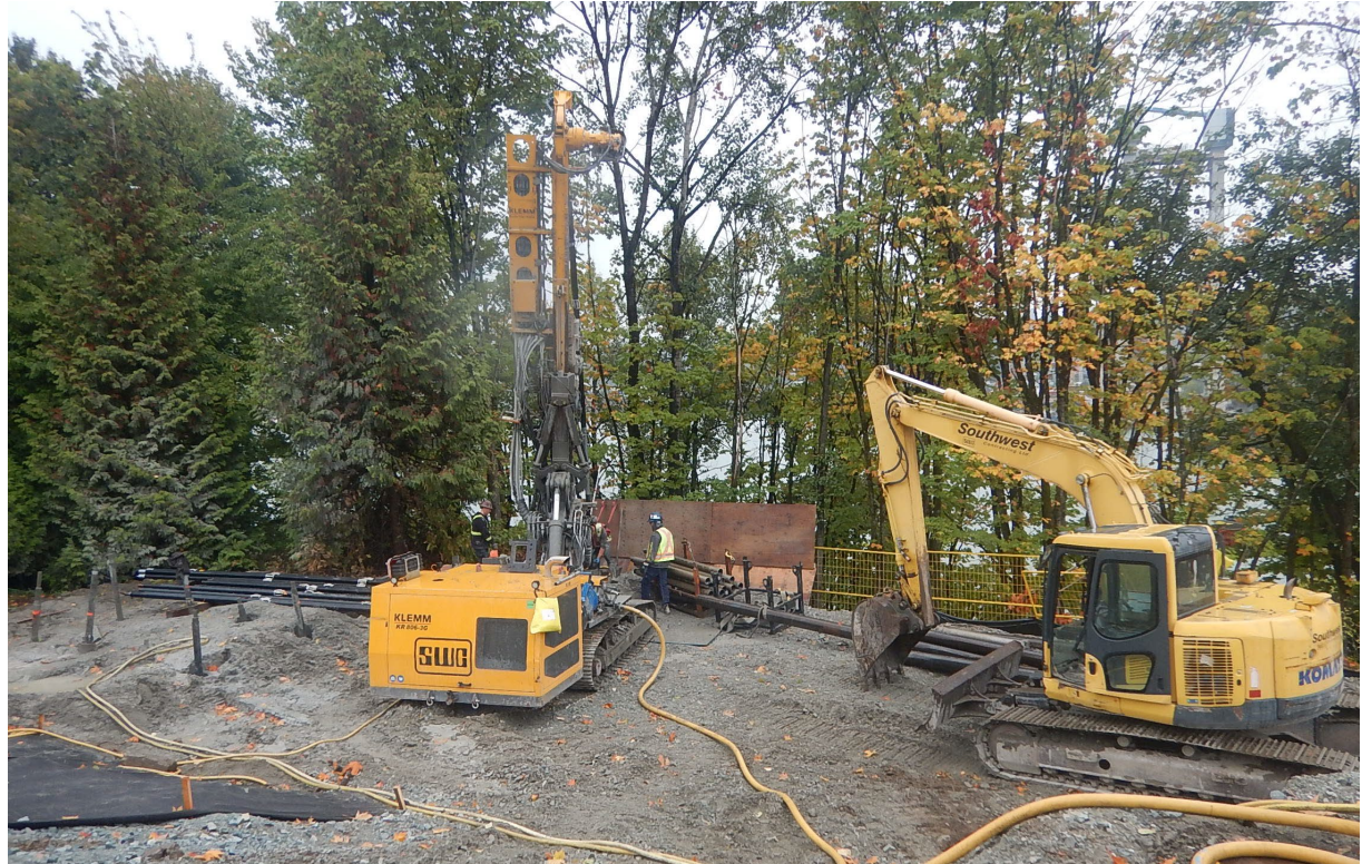
FIGURE 4 – CONSTRUCTION IS UNDERWAY ON THE NEW OVERPASS FOR THE EAST COLUMBIA MULTI-USE PATH
