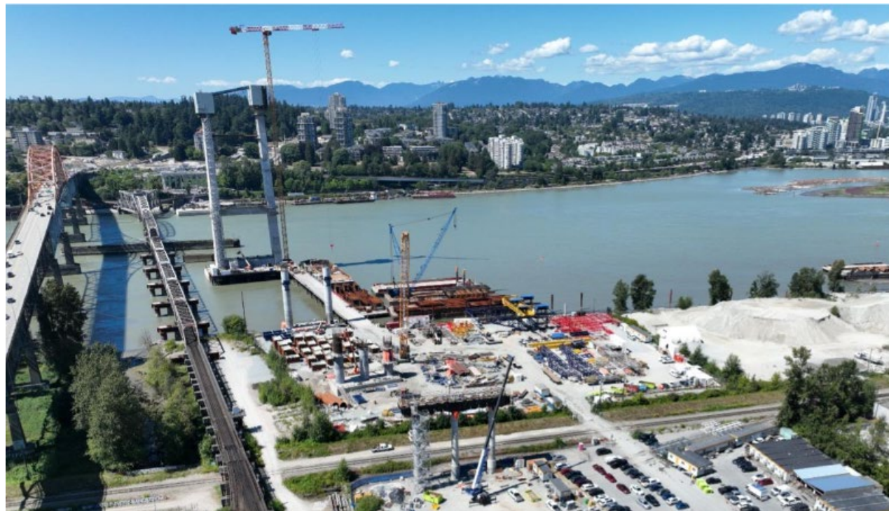
FIGURE 2 – AERIAL OF THE ONGOING S2 COLUMN CONSTRUCTION AND S3 PIER CAP CONSTRUCTION
