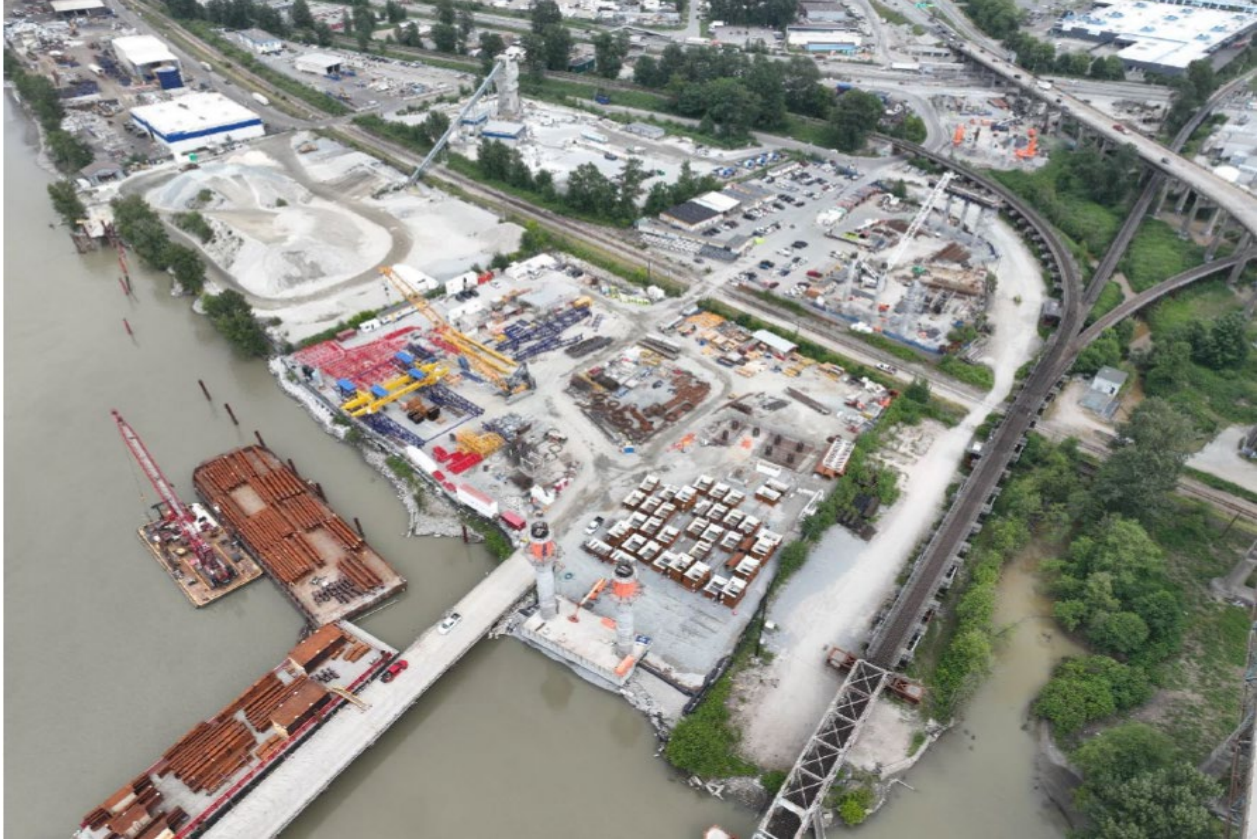
FIGURE 3 – AERIAL OF THE ONGOING FOUNDATION WORK AT S2, S3, S4 AND S5
