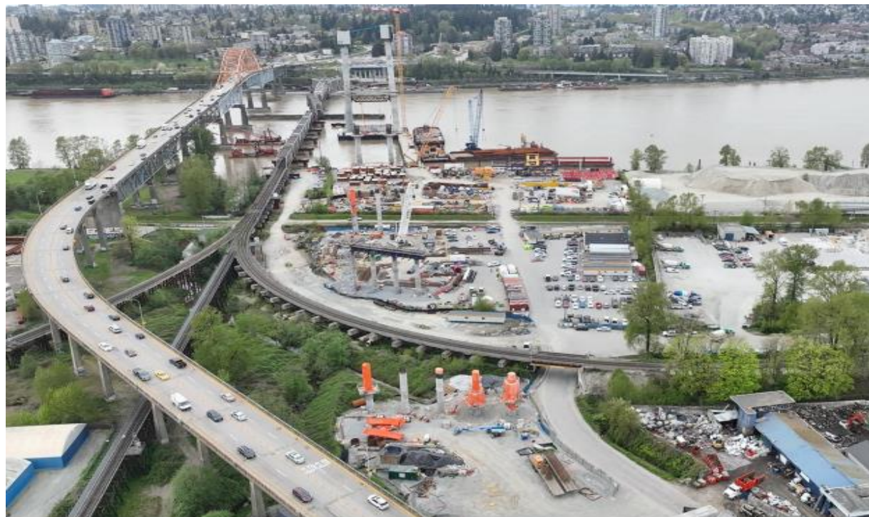
FIGURE 2 – AERIAL OF THE ONGOING COLUMN AND PIER CAP CONSTRUCTION FROM PIER S6 TO THE S1 TOWER
