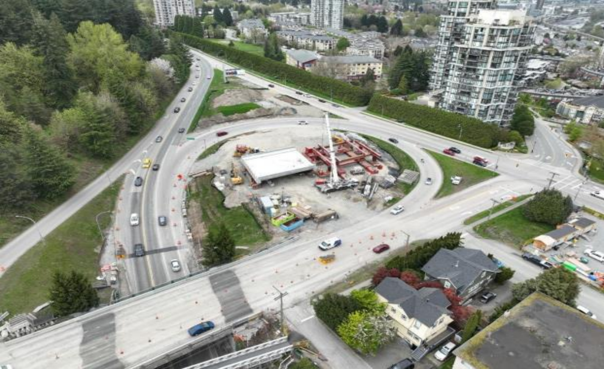
FIGURE 4 – AERIAL OF THE ROYAL AVENUE LAY DOWN AREA SHOWING THE ONGOING PREP ACTIVITIES FOR THE ROYAL AVENUE DECK REPLACEMENT WORK
