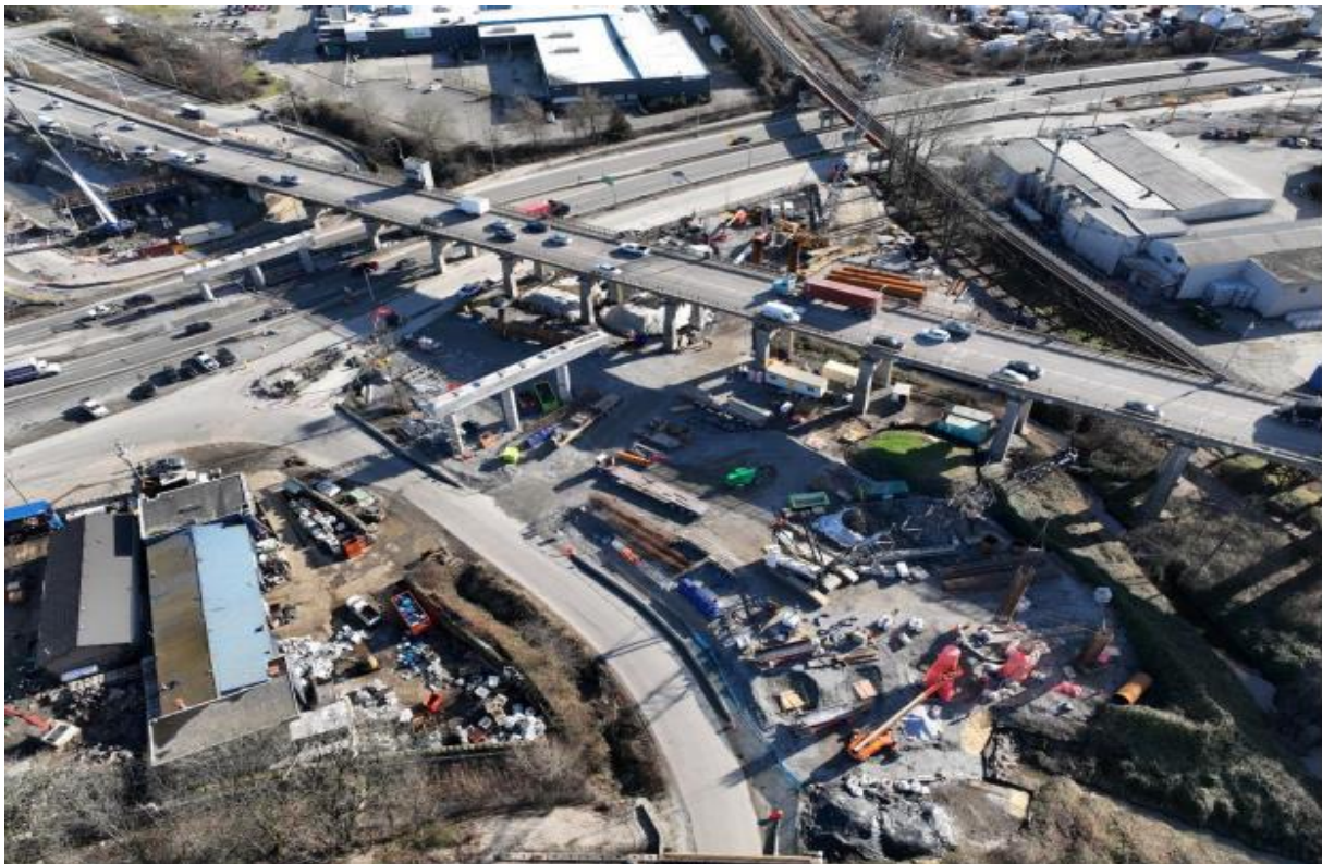
FIGURE 4 – AERIAL OF S6 COLUMN CONSTRUCTION, AND S7 PIER CAP CONSTRUCTION – SR2 PILE INSTALLATION UNDERWAY
