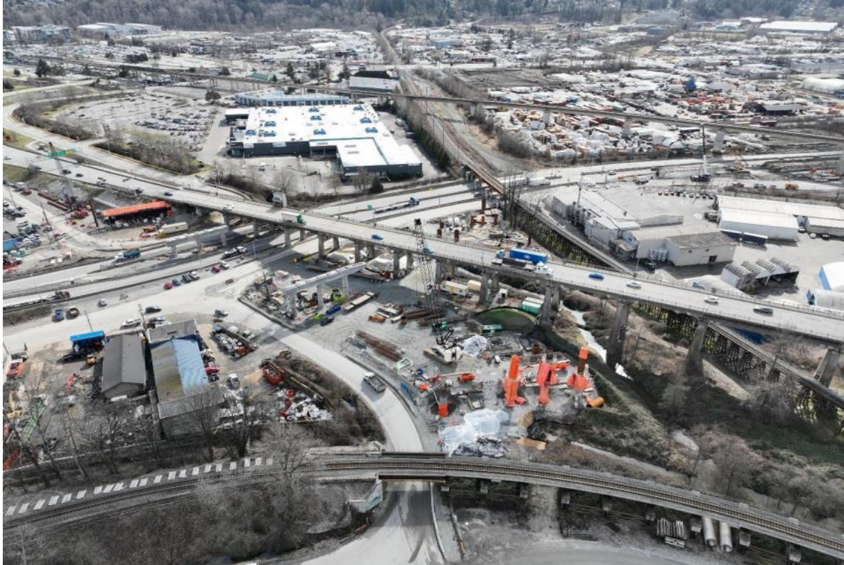
FIGURE 4 – AERIAL OF THE S6 COLUMN CONSTRUCTION, S7 PIER CAP CONSTRUCTION, AND ONGOING WORK AT SA, SR1, AND SR2
