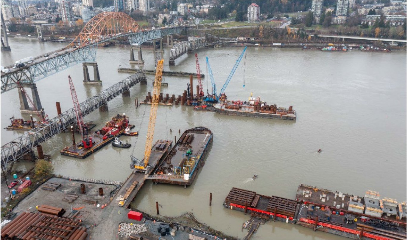
FIGURE 3 – PILE INSTALLATION AT PIER S2 (BOTTOM LEFT) AND PIER S1 (TOP MIDDLE)
